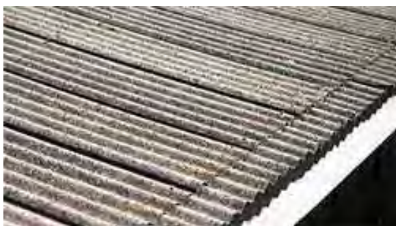
Corrugated asbestos cement sheet as roofing material for roofs of Gaushala is most preferred
